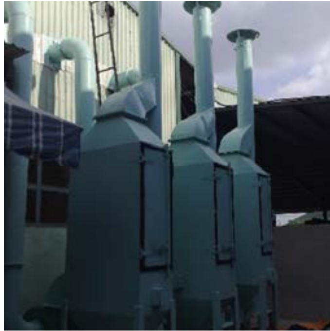
Factory dust extraction system
