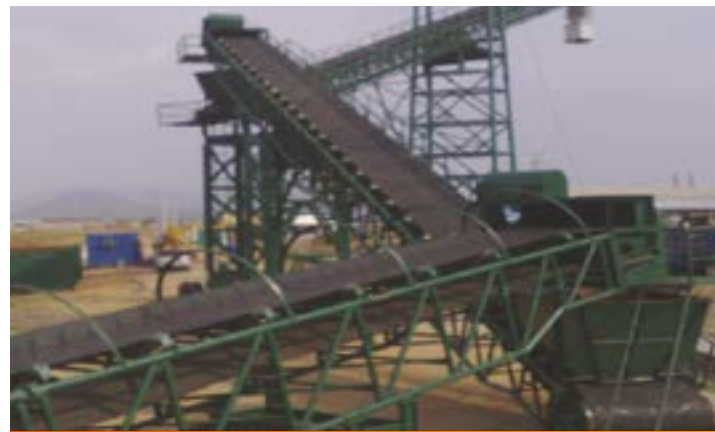
MACHINERY MECHANICAL EQUIPMENT
