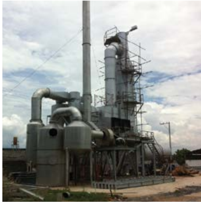
Hazardous waste incineration station
