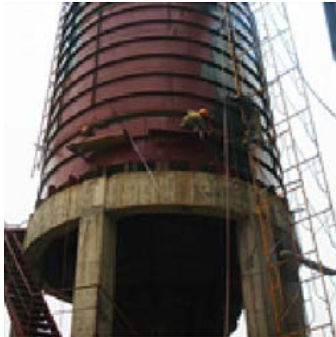
Exhaust treatment system
